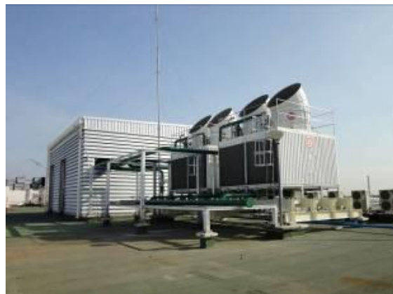
Freezing machine room with cooling tower for air-conditioning
